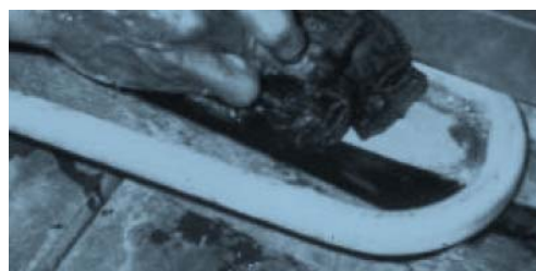
Then cool down the solder joint of pipe and sheet with damp cloths and next to remove the superfluous soldering flux
