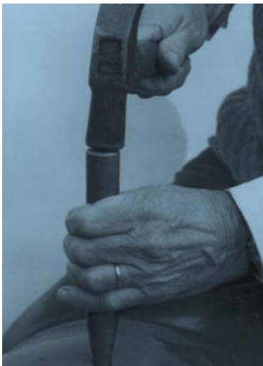
By using the steel cone and hammer widen one hole until a 1/2" piece of pipe fits in
