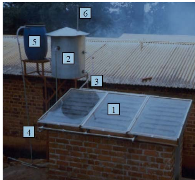
Complete solar water system
